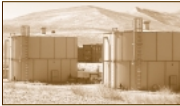
Leachate, the liquid produced by decomposing waste in a landfill, is usually collected in tanks such as these and treated. In bioreactor landfills, leachate would be used to enhance the natural breakdown of garbage.
